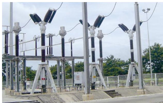
Figure 2 High voltage circuit breaker (80142C).
