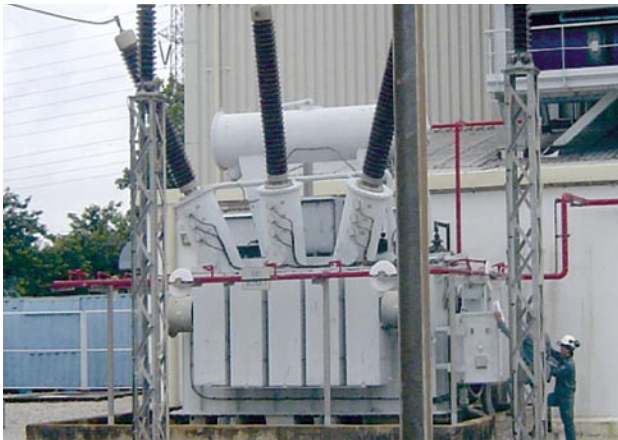
Figure 3 The station service transformer (KT2B).
